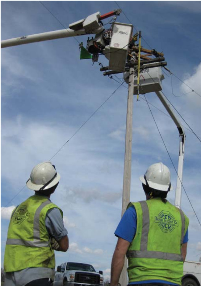
Utility workers from Chattanooga, Tennessee, help their neighbors in Fulton, Kentucky recover from the January 26th ice storm by replacing numerous power poles. At the disaster's peak, more than 700,000 customers lost power. The lack of power inhibited these customers' ability to utilize everyday communications, such as landline telephones, in order to relay any need for help or supplies. (Photo by Dianna Gee/FEMA)
